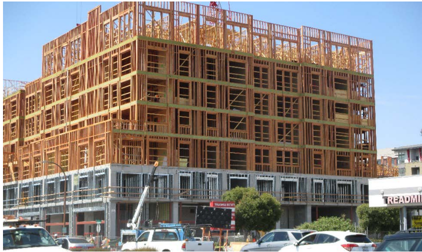
FIGURE S.0.1-1 Hybrid Construction; the Concrete Slab Supports Light Framing Superstructure (P1084)
